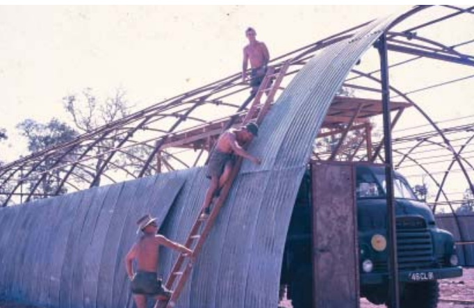
Spr s Harry Atkinson, Dennis Fitzhenry and Darryl Hess sheeting the first Romney hut with the aid of a 'mobile scaffold' constructed on the tray of a 3 ton Bedford.
