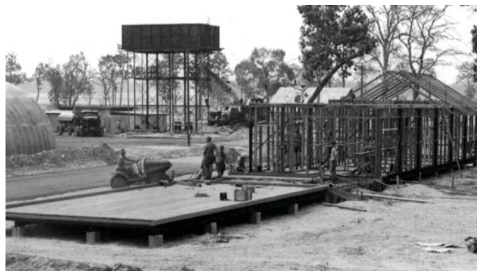
Partially-completed MRS and hospital building with the Braithwaite tank and one of the Romney huts in the background.
