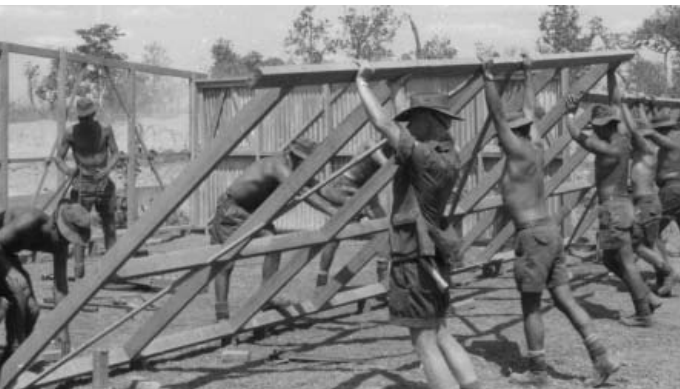
Erecting the prefabricated wall-section of the FAMTO store requires a solid team effort.
