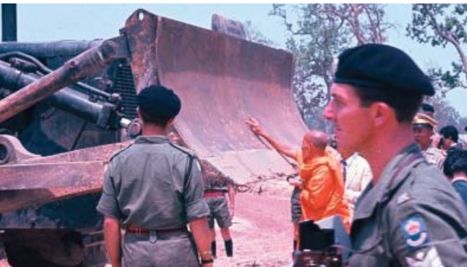
A Buddhist Monk blesses the Cat D8 before the sod-turning ceremony marking the official beginning of Operation Crown.
