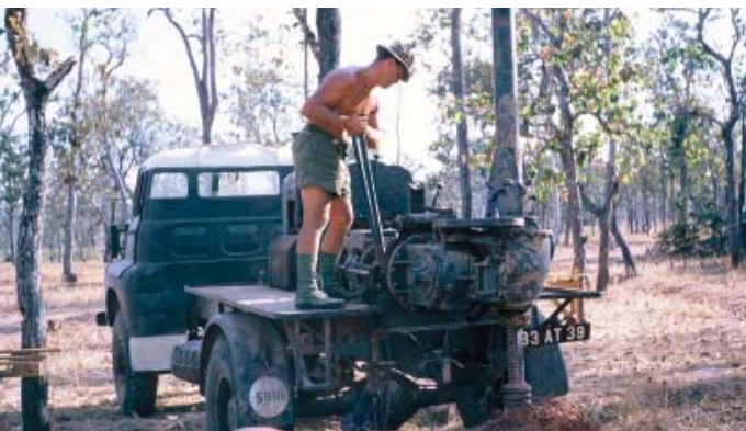
A 'Pengo' (large-diameter post-hole digger) on loan from the RAF, drilling holes for the latrines.
