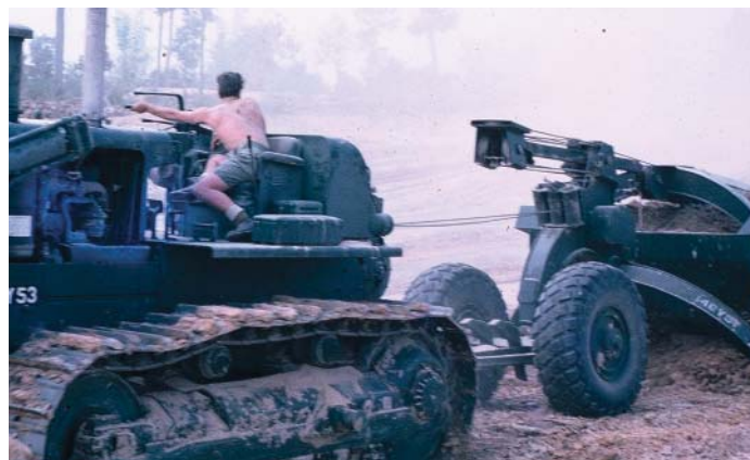
Cat D8 and open bowl scraper of 54 Field Park Sqn taking material from the borrow pit for placement on the construction site and helipad.
