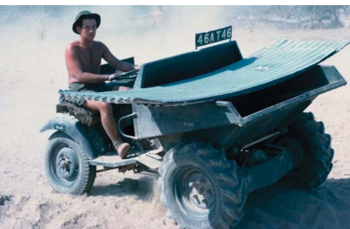
Spr Ian Tibbles delivering cladding for a Romney in a Rough Rider motorised skip, complete with accompanying dust.
